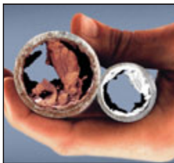
Hard water produces a scaly buildup which can clog pipes and appliances.
